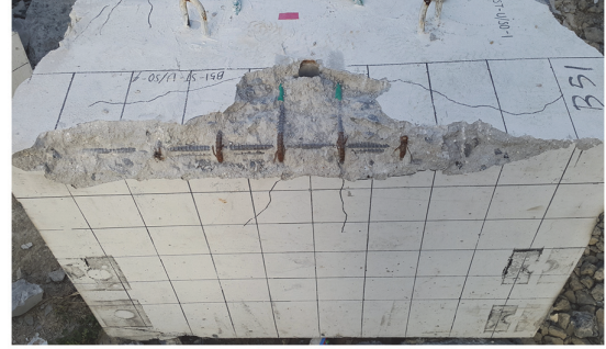
Fig. 14. Scene after removal of fractured concrete cover (ST-U/S0-4)
