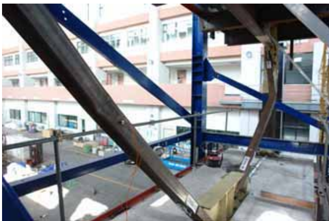
Fig. 10 Out-of plane buckling of 2 nd floor braces
