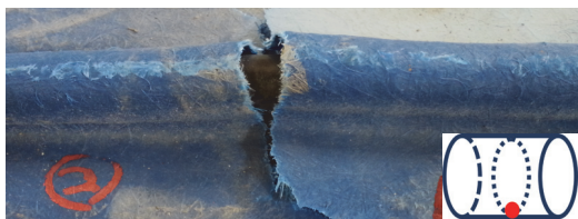
(b) Type A: sheath fracture in the steel pipe ring
