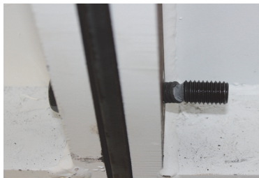
Failure of H.T.B
