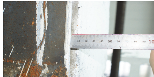
(d) Sliding between concrete and steel
