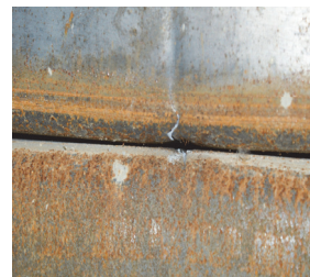
(a) Crack of Z-shaped side plate
