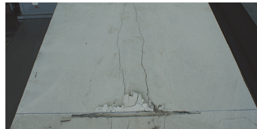
(c) Longitudinal crack of concrete slab
