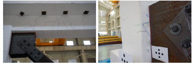
(a) Upper beam (b) Drop out of concrete
