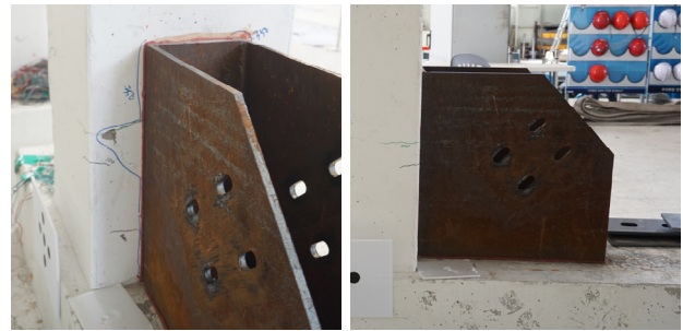
Fig. 11. Rusty surface of damper part
