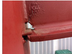
(e) Weld fracture
