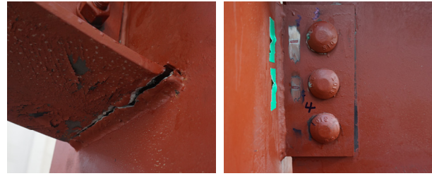
(a) Weld fracture
